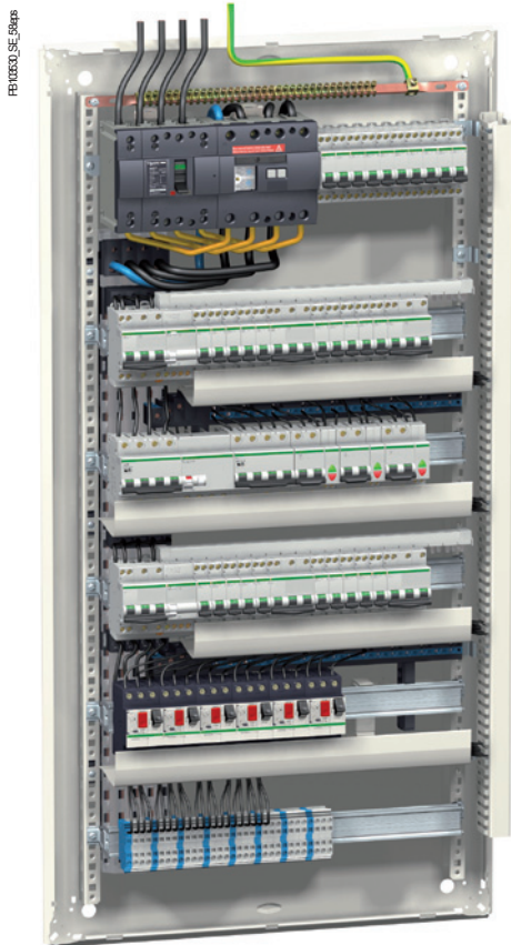
NG160 in modular enclosure.
